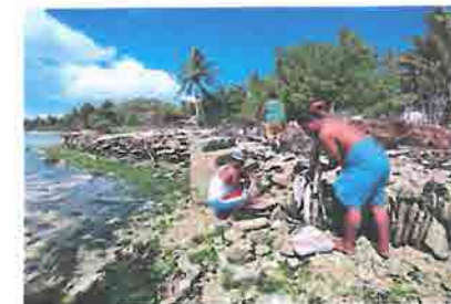
People of the Pacific ocean island of Kiribati building a stone wall against rising sea levels. Poorer countries will bear the brunt of climate change. – AFP
